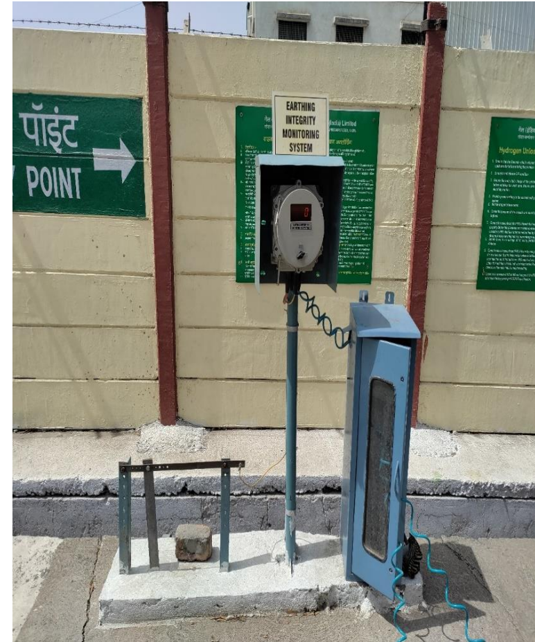
Earthing Integrity monitoring system for Cascade which is connected with PLC to ensure continuity
