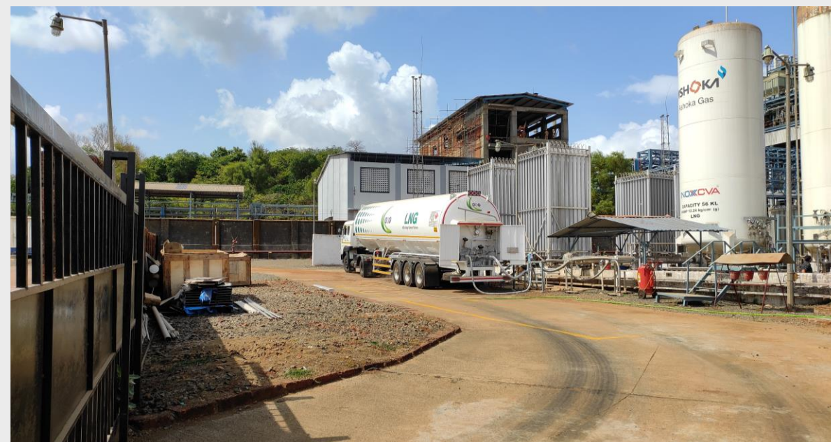
Safely reach at LNG/LCNG station and unloading
